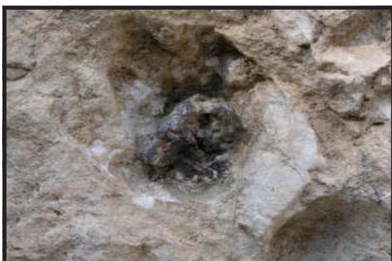
Close-up view of iron pin embedded deeply into the rock by melted lead.
